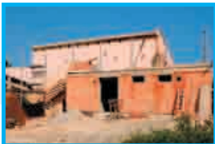
Rozestavěná přístavba pavilonu žiraf The additional building of the house of giraffes during it is construction
