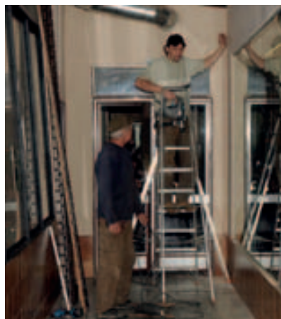
Opravy stropu v pavilonu opic Repair of the ceiling of the monkey house
