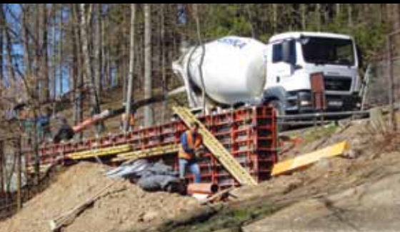
Stavba opěrné zdi u safari /Construction of retaining wall in the safari area/
