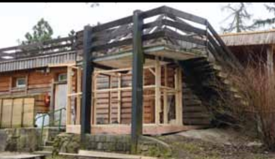
Stavba skladu u gastro provozu /The construction of a storage near our gastro services/
