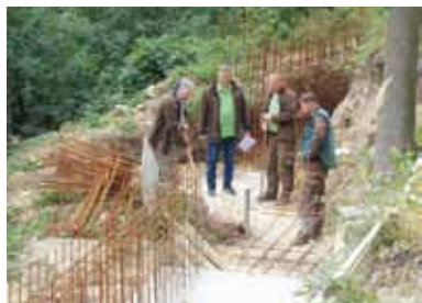
Stavba opěrné zdi u safari /Construction of the support wall in the safari area/
