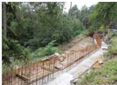
Stavba opěrné zdi u safari Amerika /Constructing the support wall at the Safari/
